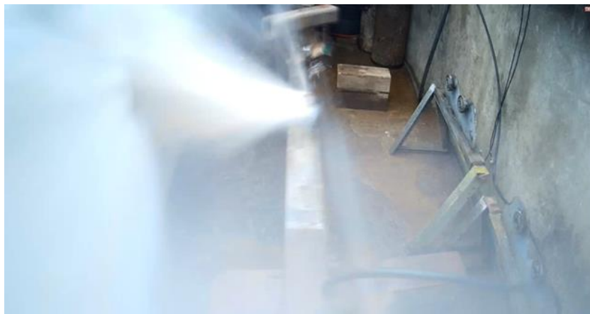
Fig. 16. The Y6 pipeline section at the moment of its failure.
