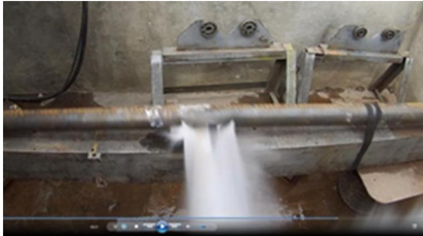
Fig. 15. The Y3 pipeline section at the moment of its failure.
