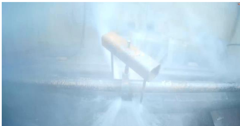
Fig. 17. The Y8 pipeline section at the moment of its failure.
