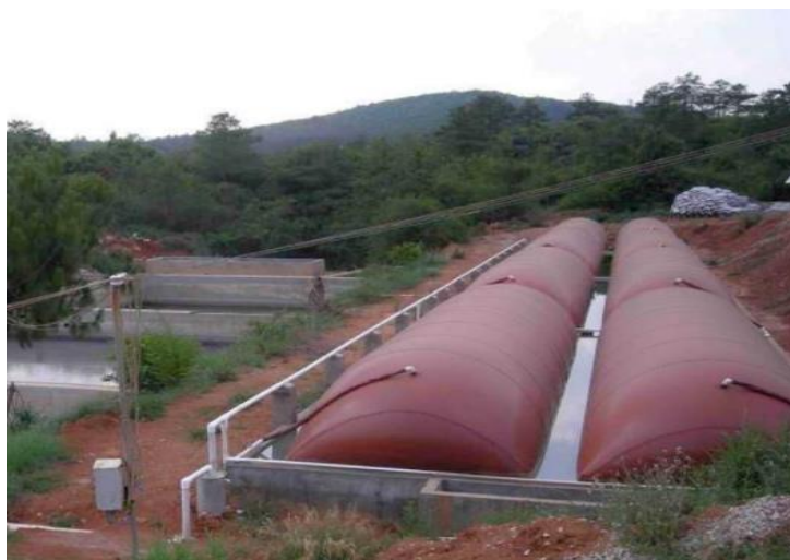
Figure 47. Balloon types biogas plant.
